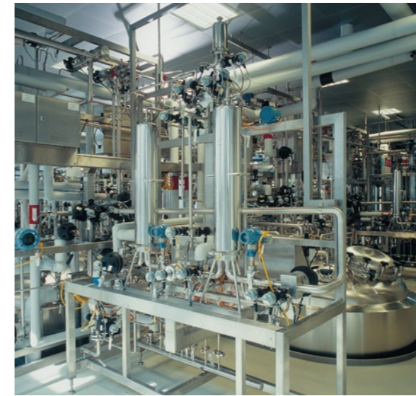
Fermentation plant (Fermentation skid)
